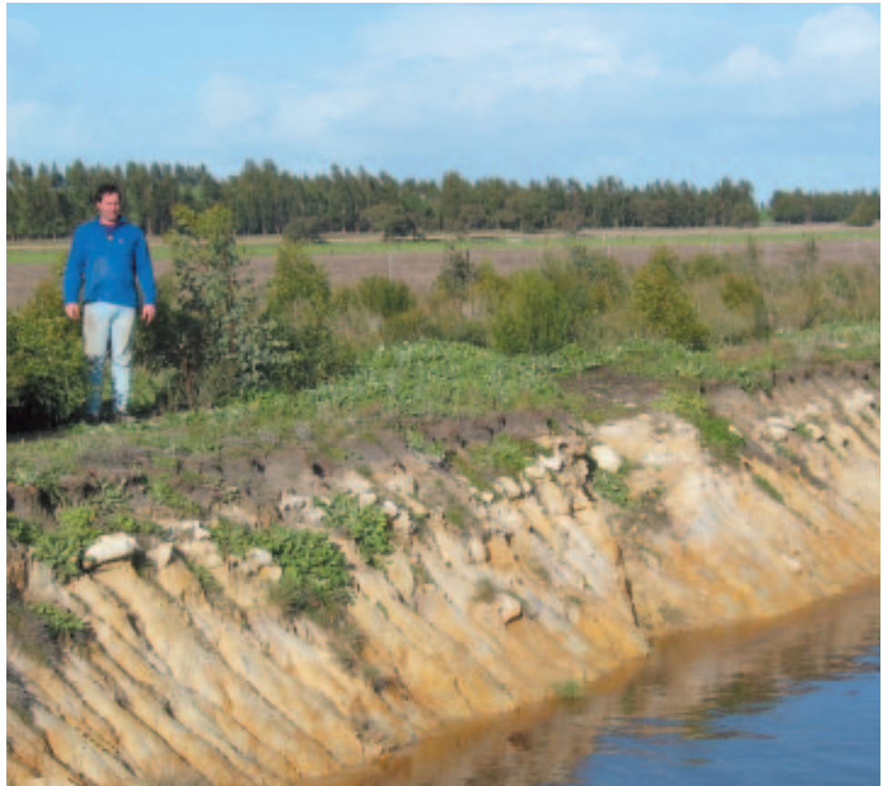
Above: Deep drains have relieved the impact of rising water tables but introduced soil management challenges.
