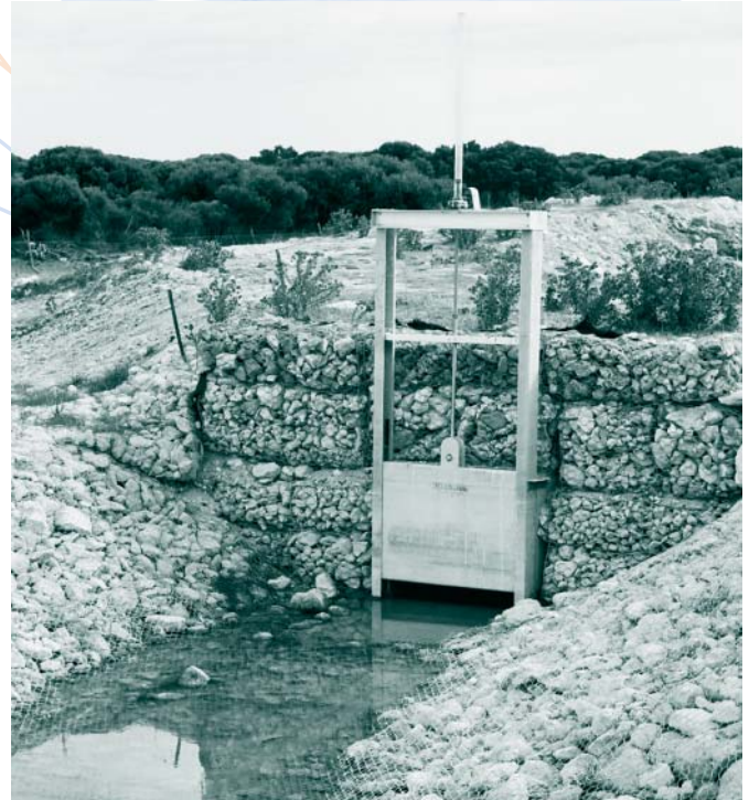
Flow control gate installed to manage water movement along a drain
