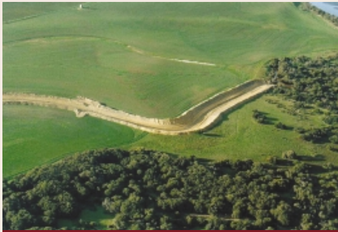
An aerial view of a section of the Cummins Wanilla drainage project showing the graded longitudinal curve. For the implementation of successful drains a detailed site plan must be drawn up which shows curve details which can then be pegged out prior to excavation.
