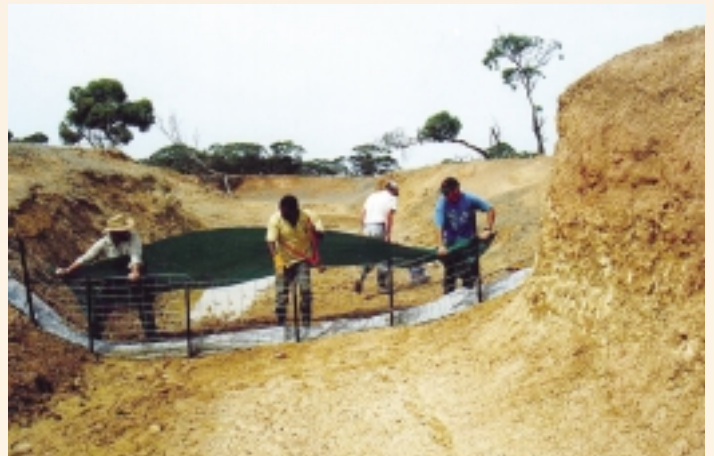
Grade control structure being installed as part of the Cummins Wanilla Drainage Scheme. Such structures help slow water flow where mean fall is too great. A fall of no more than 0.7: 100 is desirable.
