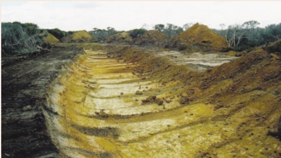
A large surface drain developed as part of the Cummins Wanilla drainage project 1999. (Note that the sides have been battered to a 3:1 slope) Slope battering reduces erosive conditions which could cause slumping of the sides. The steepness of the batter depends upon the soil type, generally the more potentially erosive the soil the more gently graded the profile. The long sinuous curve in the drain reduces potential erosion of the drain in high rainfall events. Such curves should always be included in drain design to mimic natural stream flow patterns.
